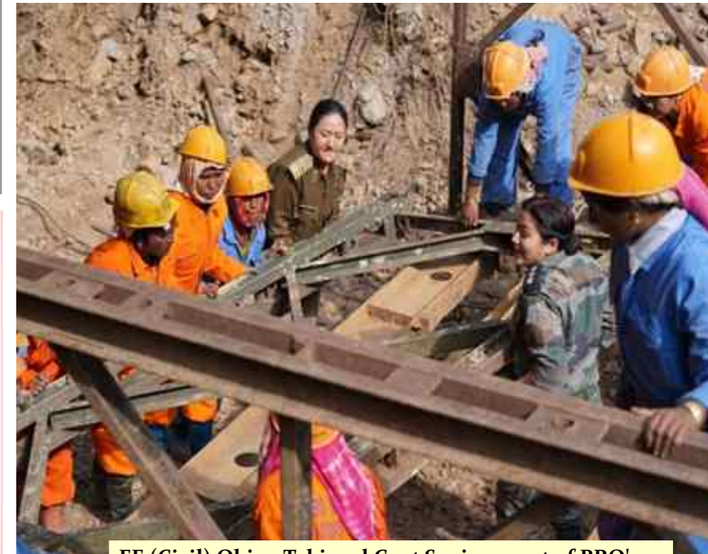
EE (Civil) Obing Taki and Capt Sania as part of BRO's All Women Team de-launching a Bailey Bridge in Arunachal Pradesh
