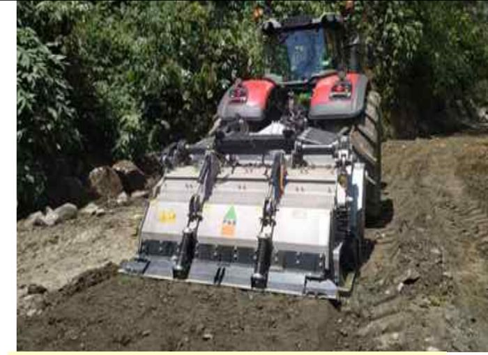
Construction of Cementitious Base Course on TCC-Taksing and TCC-Maza Roads in Arunachal Pradesh
